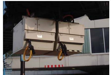
Dual coils mounted under a passenger bridge.
