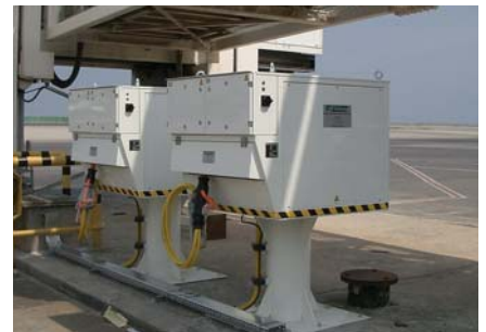
Specialised cable coils at Nice Airport.
